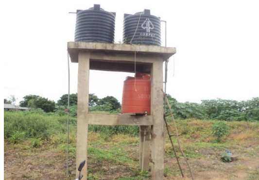
Plate 1a: Provision of Water tanks attached to borehole in Tede community
