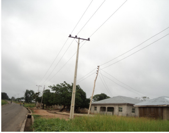
Plate 2: Electricity supply in Sepeteri community
